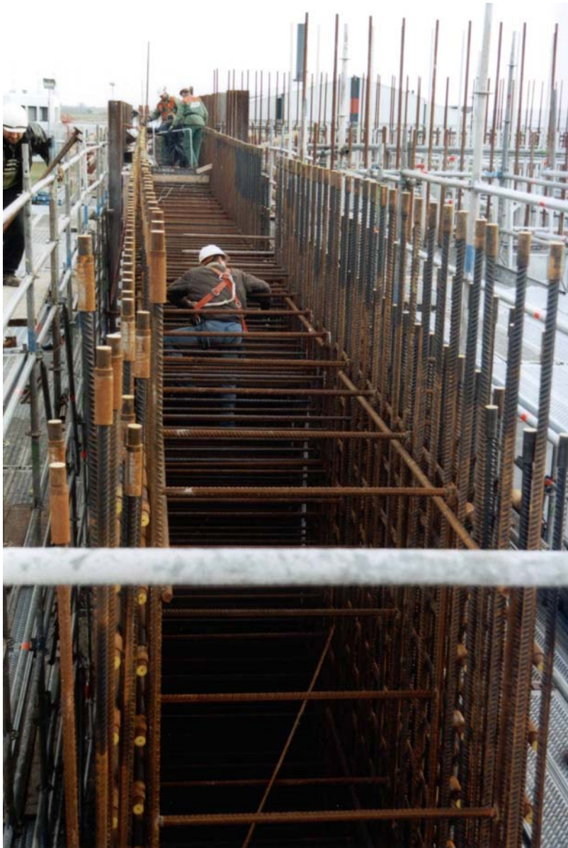
Figure A.5. Worker in the concrete at work in 1,7 meter thick outer wall.
