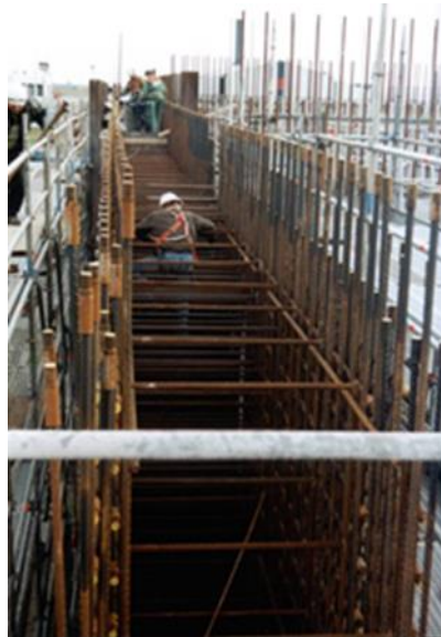
Figure A.5 Worker at work in a concrete 1.7 m thick outer wall
